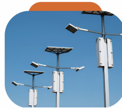
Solar Street lights
